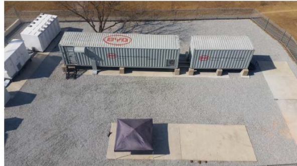
- Eskom battery testing site in Rosherville, Pretoria
