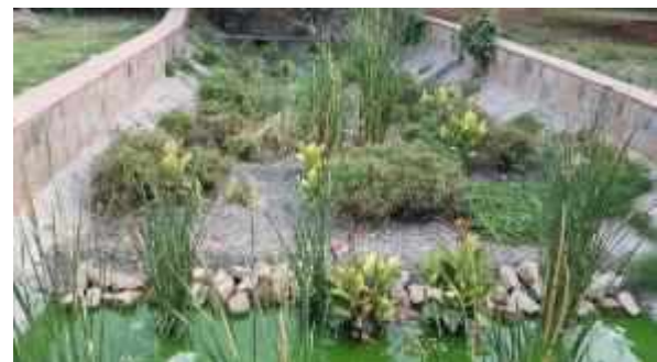
Figure 10 – Outfalls Conversion of a drainage canal into a subsurface flow constructed wetland
