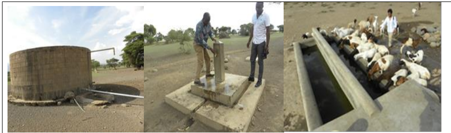
Water storage tank, water delivery points (DPs) and cattle trough in Irerendeni Village, Engaruka
