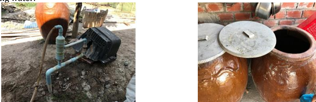
Figure 3. Intake pump for ground water / Rain water storage
