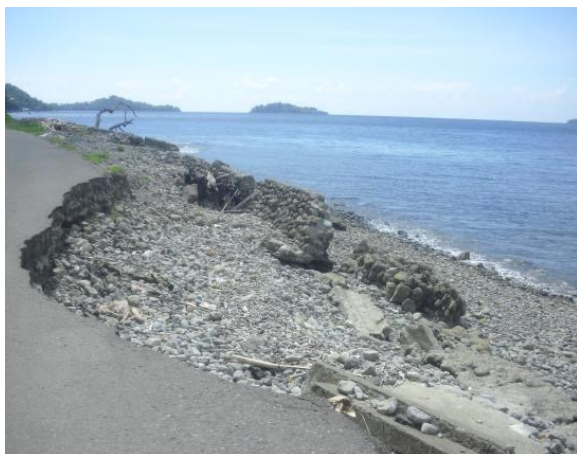
Figure 2. The impact of tidal waves and abrasion in the form of damage to road infrastructure and breakwater walls due to tidal waves
